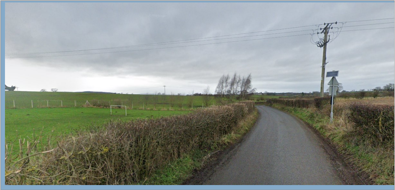
Figure 3 Existing powerlines above the playing field and utility pole on side road
